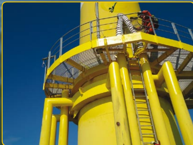
Phase 1 refurbishment to walkway and underside of monopile complete. Phase 2 will take monopile refurbishment from underneath top collar section below grating down to sea level.
