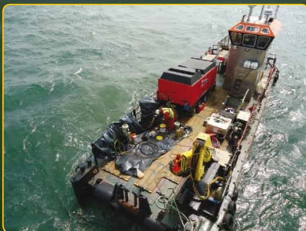
Workboat alongside monopile carrying all necessary tools and equipment to perform blasting, coating and mechanical works.
